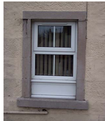
Poor window replacement
