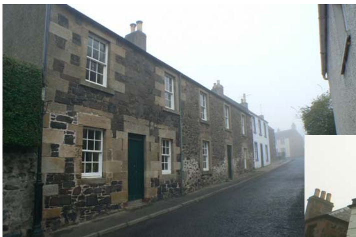
A terrace of good quality local vernacular buildings; whin rubble built with blonde sandstone dressings
