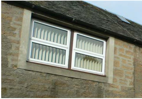
Alterations to window fenestration and inappropriate window replacement
