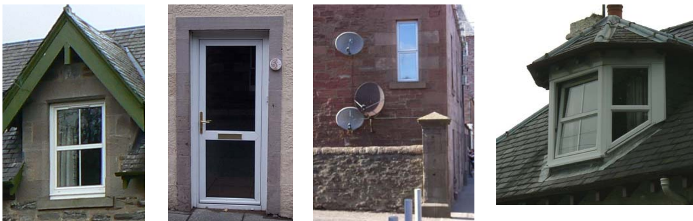
Examples of permitted development, thus allowing erosion of original features and visual jarring
