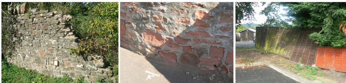
Examples of boundaries within the conservation area which are in need of repair or enhancement.
