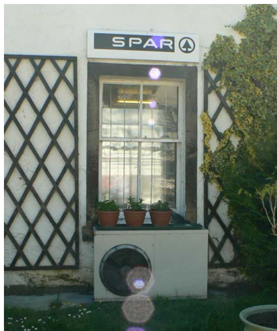
Air conditioning unit in garden ground of Post Office
