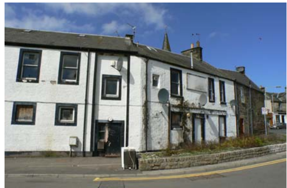
Public house in poor condition
