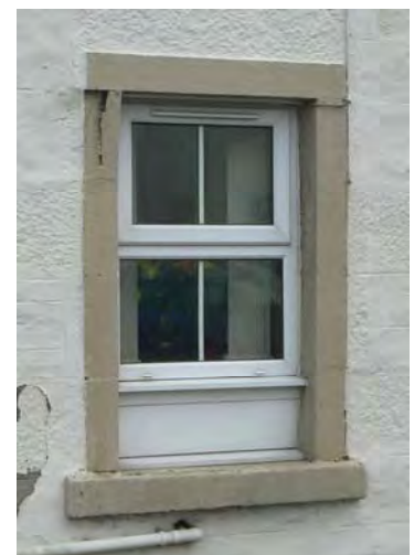
Right, an example of an inappropriate replacement window
