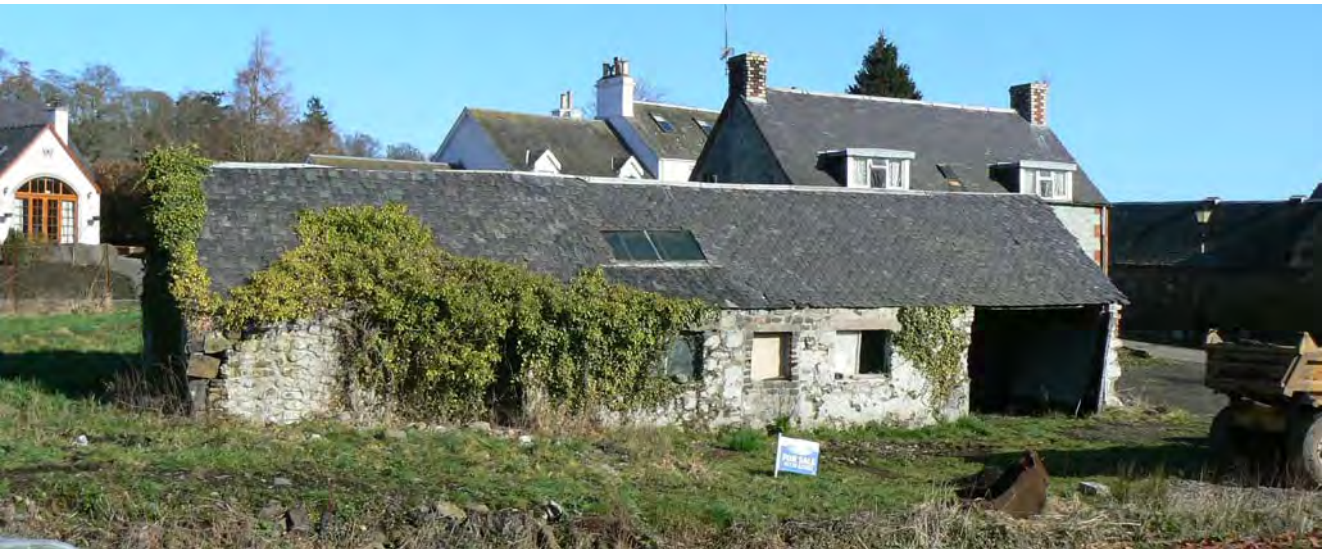
Former Smithy now a building at risk
