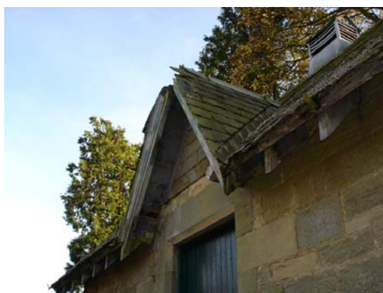
Rotting timbers at the Wash House
