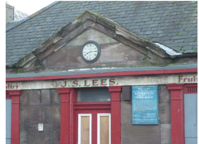
Old Toll House - may be candidate for Historic Building funding
