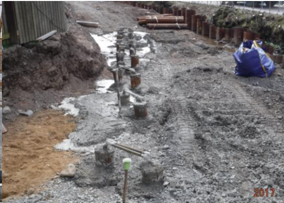
34. Lochty Park – completion of tubular piles. This will form the foundation for the new flood wall.
