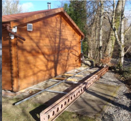
11. Craigneuk – relocation of summer house to allow construction of the flood wall.
