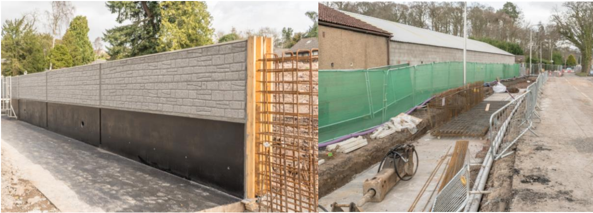
28. Trout Farm – completion of reinforced concrete flood wall with aesthetic stone finish (black area will be below ground).
