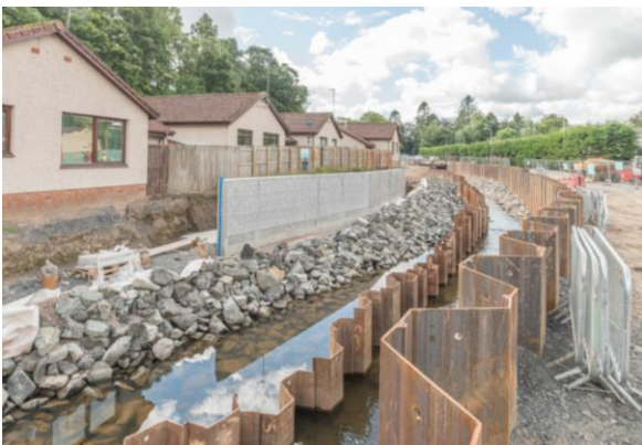
53. Lochty Park – Erosion protection complete with concrete flood walls behind. Temporary sheet piles in the burn and permanent piles to the right.
