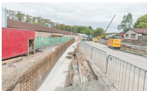
40. Lochty – construction of retaining wall reinforcement. (This is required in order to raise the road here).
