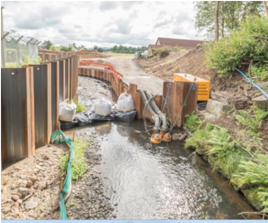
51. Puddledub – temporary damming of the East Pow Burn to allow dry working area. Water pumped forward.
