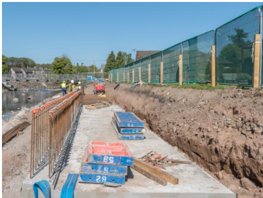
35. Deer Park – looking upstream at new flood wall bases and stem reinforcement.
