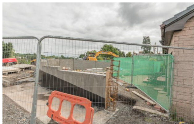
48. Brockhill – completed retaining wall at front of Brockhill. This is required to accommodate access roads for the raised Confluence Bridge.
