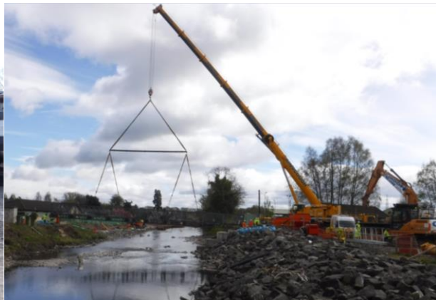
31. Black Bridge – temporary relocation of Black Bridge in order to construct new bridge.
