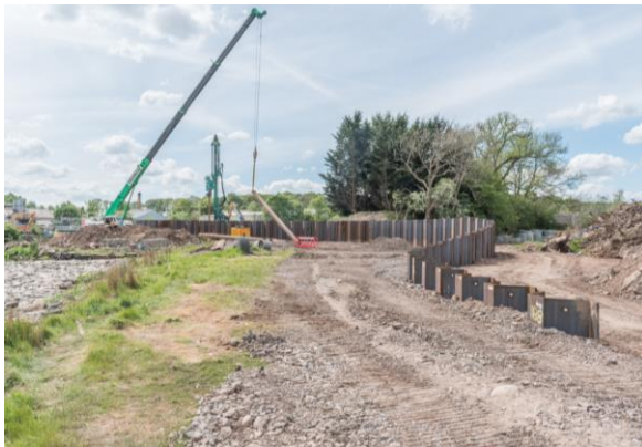
43. Low's Weir – installation of sheet piles. The piles will be hidden under a flood embankment.
