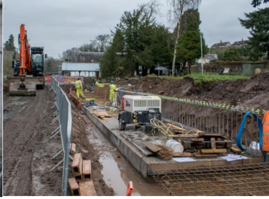
17. Trout Farm – flood wall concrete base complete and reinforcement erected for subsequent bases.
