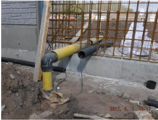
33. Druid House – Not all services can be relocated away from the new flood wall. Some have to be designed into it.
