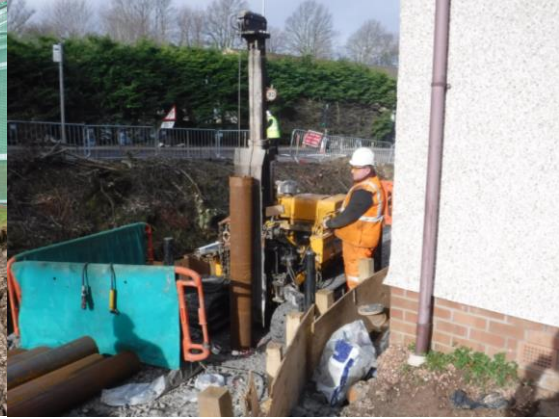
27. Lochty Park – installation of tubular piles (that will form the foundation of the new flood wall).
