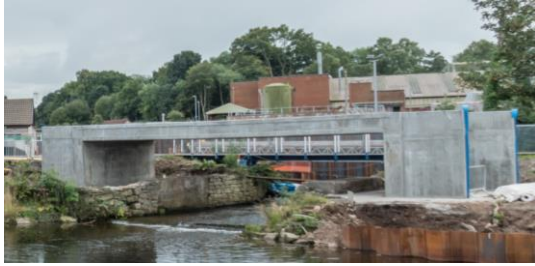
63. Confluence Bridge at Lows Works Cottages – new bridge completed, but due to a failure with the temporary support works the bridge deck sagged and had to be replaced.
