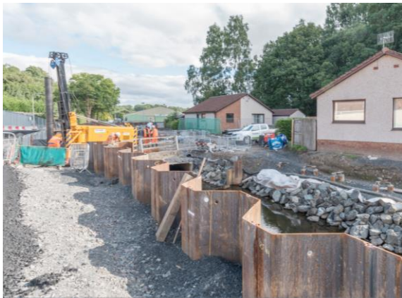
57. Lochty Park – continuation of flood walls and installation of piles for road bridge.
