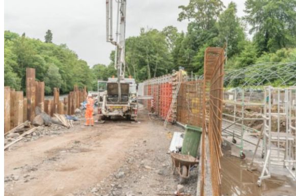
46. Trout Farm – reinforcement stem of flood wall being constructed (continuation from photo 38).
