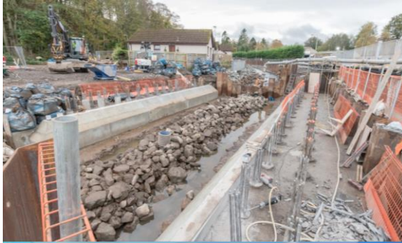
76. Lochty Bridge – ongoing construction of bridge, ready for placing the steel reinforcement for the abutments.
