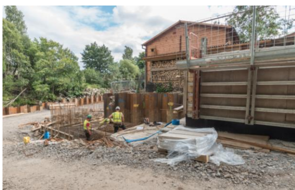
62. Craignuek – construction of flood wall (right), flood wall base (left) and temporary sheet piles to stabilise surrounding ground (rear).
