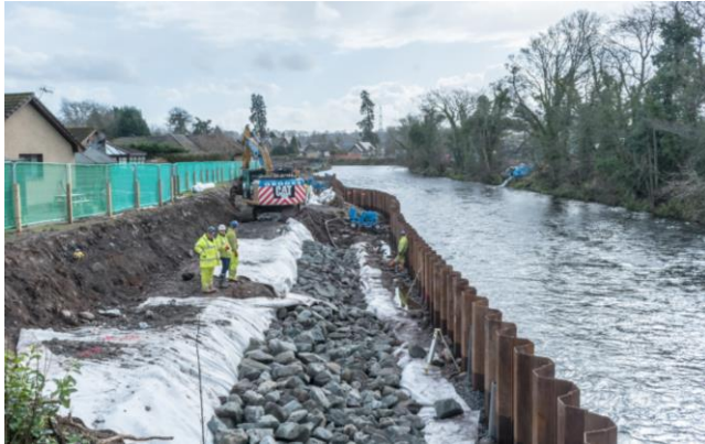
20. Deer Park – construction of erosion protection system (geotextile under with interlocking rock armour on top).
