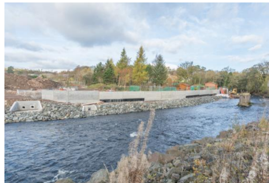
79. Craigneuk – view of ongoing works to flood wall and pumping station outfall at Craigneuk.
