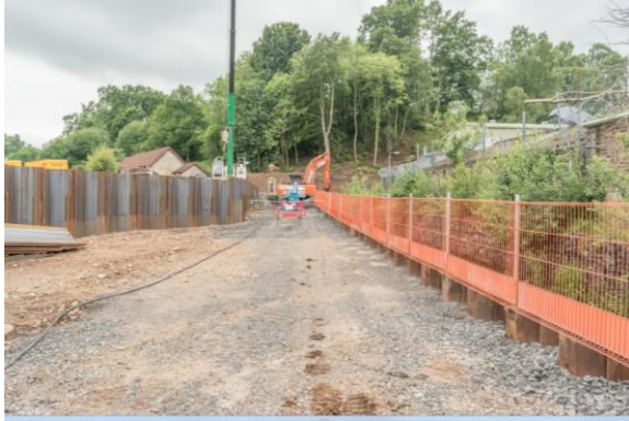
45. Puddledub – installation of sheet piles (left). Temporary sheet piles and safety rail within the East Pow Burn.
