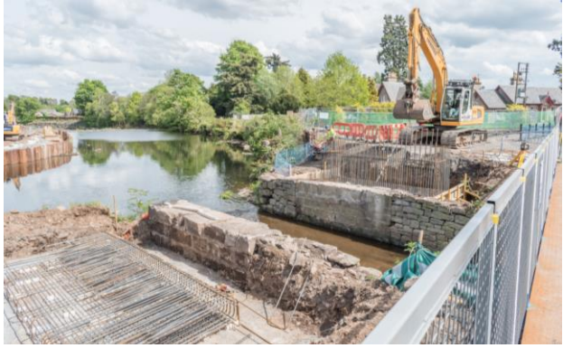
41. Deer Park – construction of Reinforcement base and stem for the new Confluence Bridge at Brockhill.
