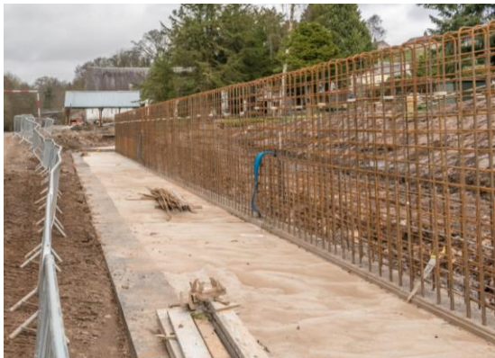
24. Trout Farm – completion of flood wall bases and erection of reinforcement for flood wall stems.
