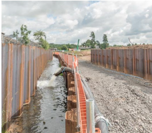
52. Puddledub – water pumped back into East Pow Burn. Permanent sheet piles to protect Vector (left) and Puddledub (right). Temporary piles in the middle.
