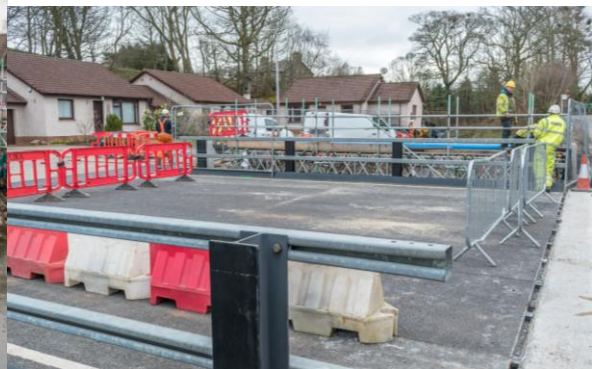
23. Lochty Park – installation of temporary bridge to allow demolition and construction of new Lochty Park bridge.
