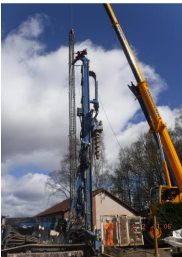
32. Lochty Park – construction of bridge piles. Lowering of steel reinforcement cage into the pile.
