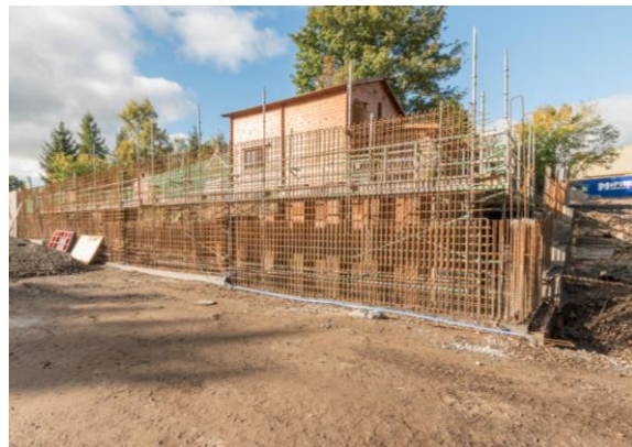
68. Craigneuk – placement of flood wall stem reinforcement prior to pouring concrete wall.
