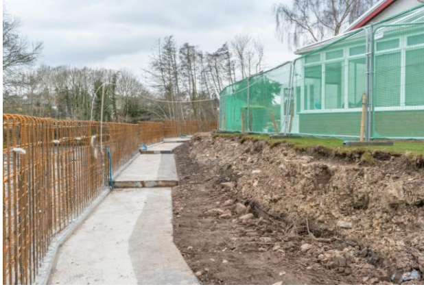
26. Druid House – completion of flood wall bases and erection of reinforcement for flood wall stems.
