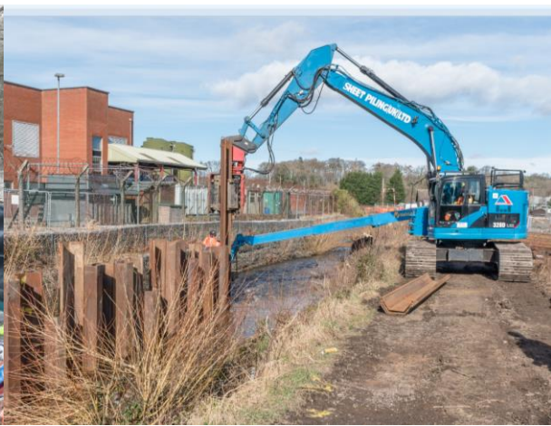
19. Puddledub – installation of temporary sheet piles in East Pow Burn for safe working and environmental reasons.
