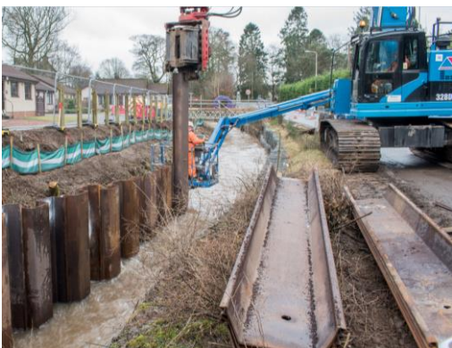
14. Lochty Park – installation of temporary sheet piles for safe working and environmental reasons.
