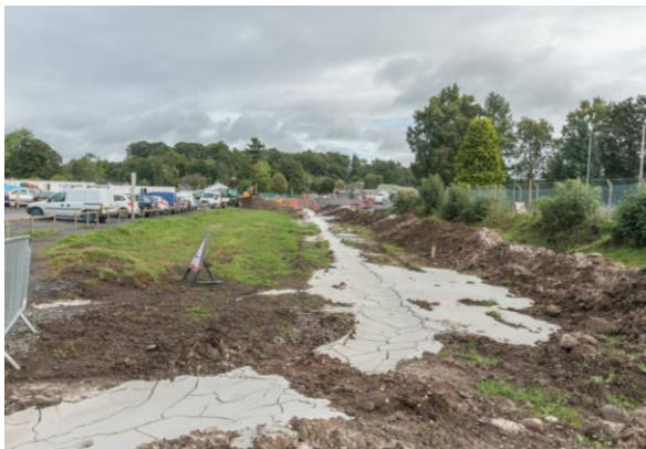
67. Cricket Pitch – linear channel of bentonite upon which the flood embankment will be erected.
