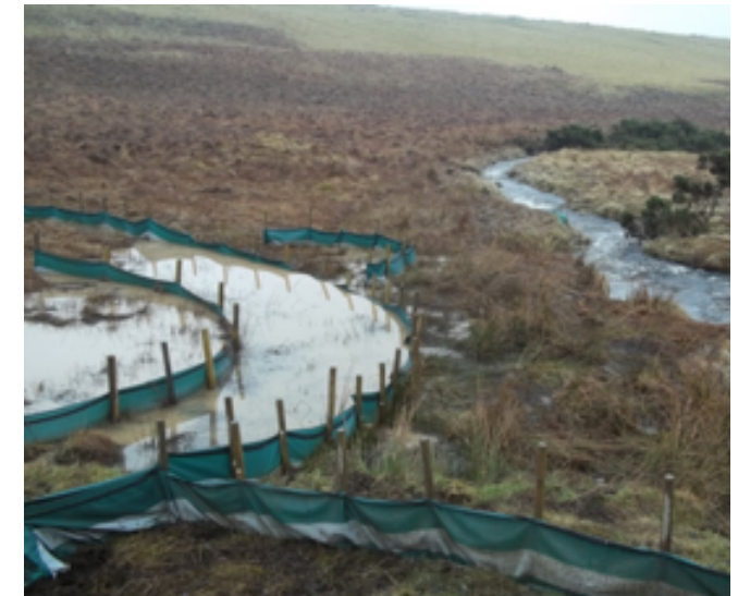
Multiple layers of silt fencing in place to prevent pollution of the nearby watercourse
