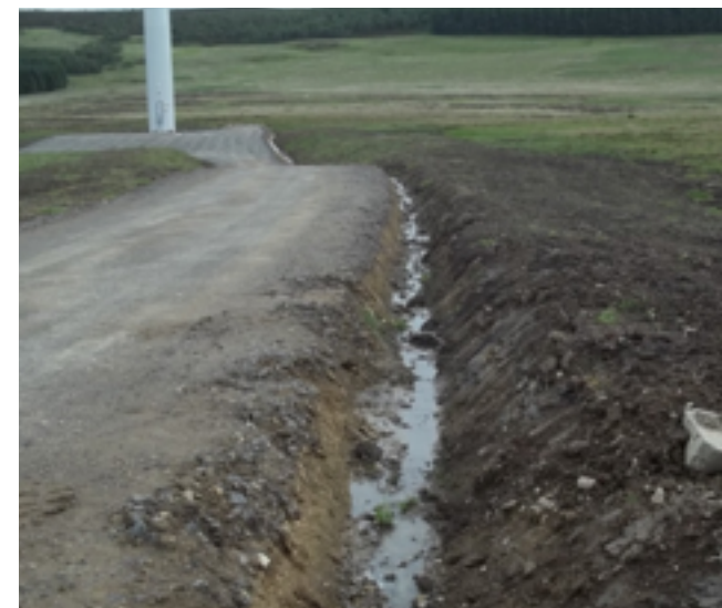
Track verge reinstatement with 'V' ditch. Check dams were requested at 10-20m intervals to slow running water and reduce scour.
