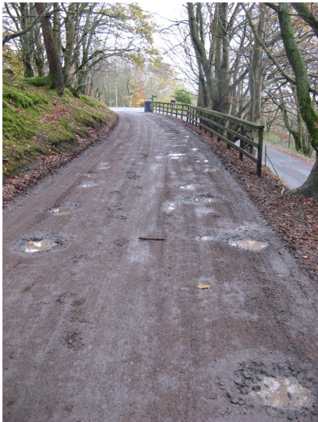
Potholes on access track to Upper Car Park
