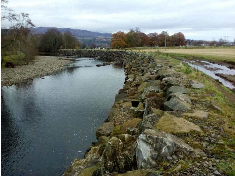
Figure 2-5: Photo taken during the site visit of the downstream reach of the Water of Ruchill (Reach 4)
