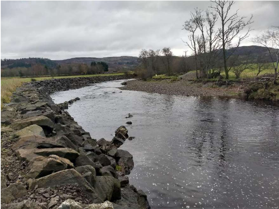
Figure 3-13: Photo of rip-rap bank protection and J-vanes at Ruchillside. A gravel bar has formed on the inside meander bend. Evidence of gravel extraction is visible on this bar.
