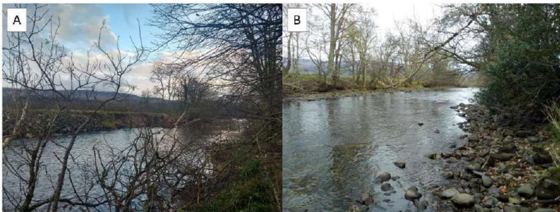
Figure 2-4: Photos of the upstream reach of the Water of Ruchill (A) Shows rip-rap bank protection on the left bank which has been out flanked at the downstream end. (B) Shows a typical stretch of the Reach 3
