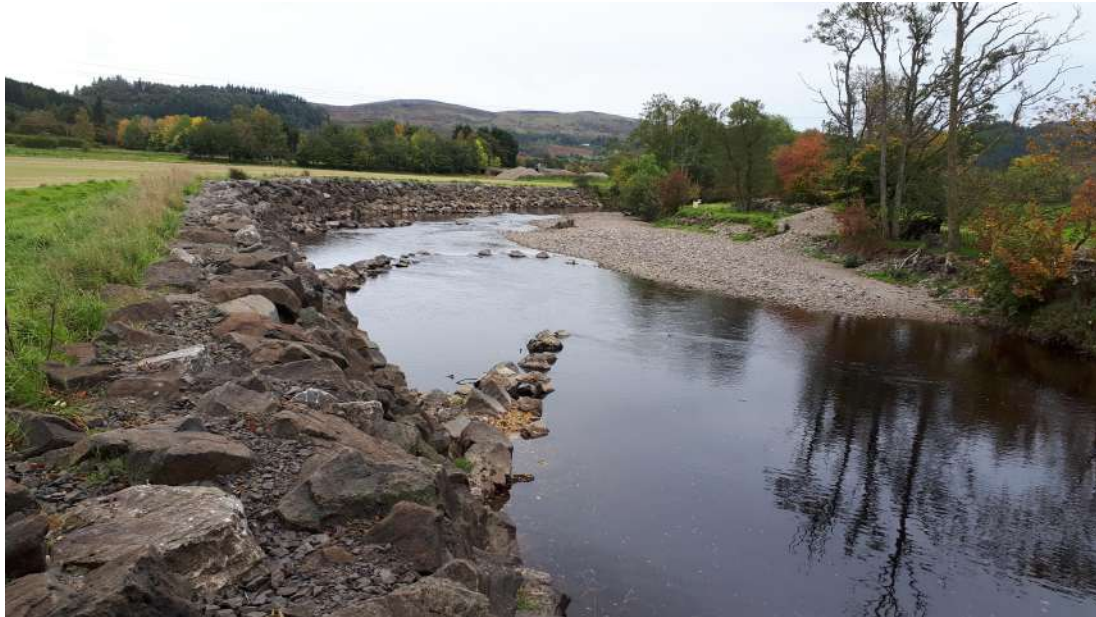
Photograph 3: Groynes and bank-side reinforcement on the Water of Ruchill. Slow water downstream of the groynes, coupled to the crevices between the rocks, was considered to be suitable for crayfish.
