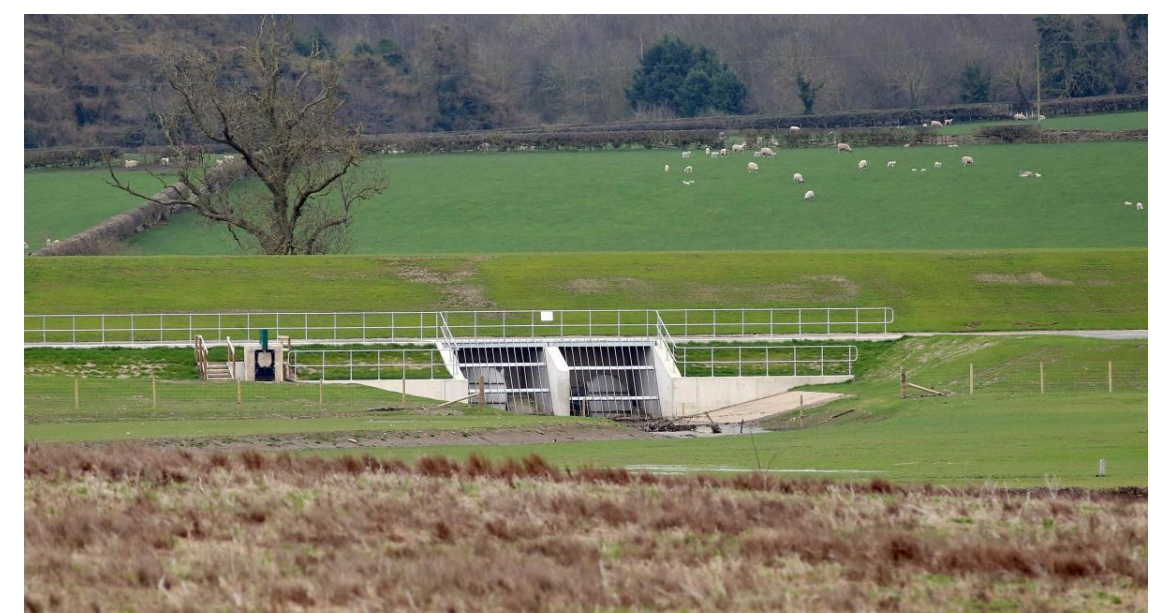
Figure 16: Example of a Control Structure
