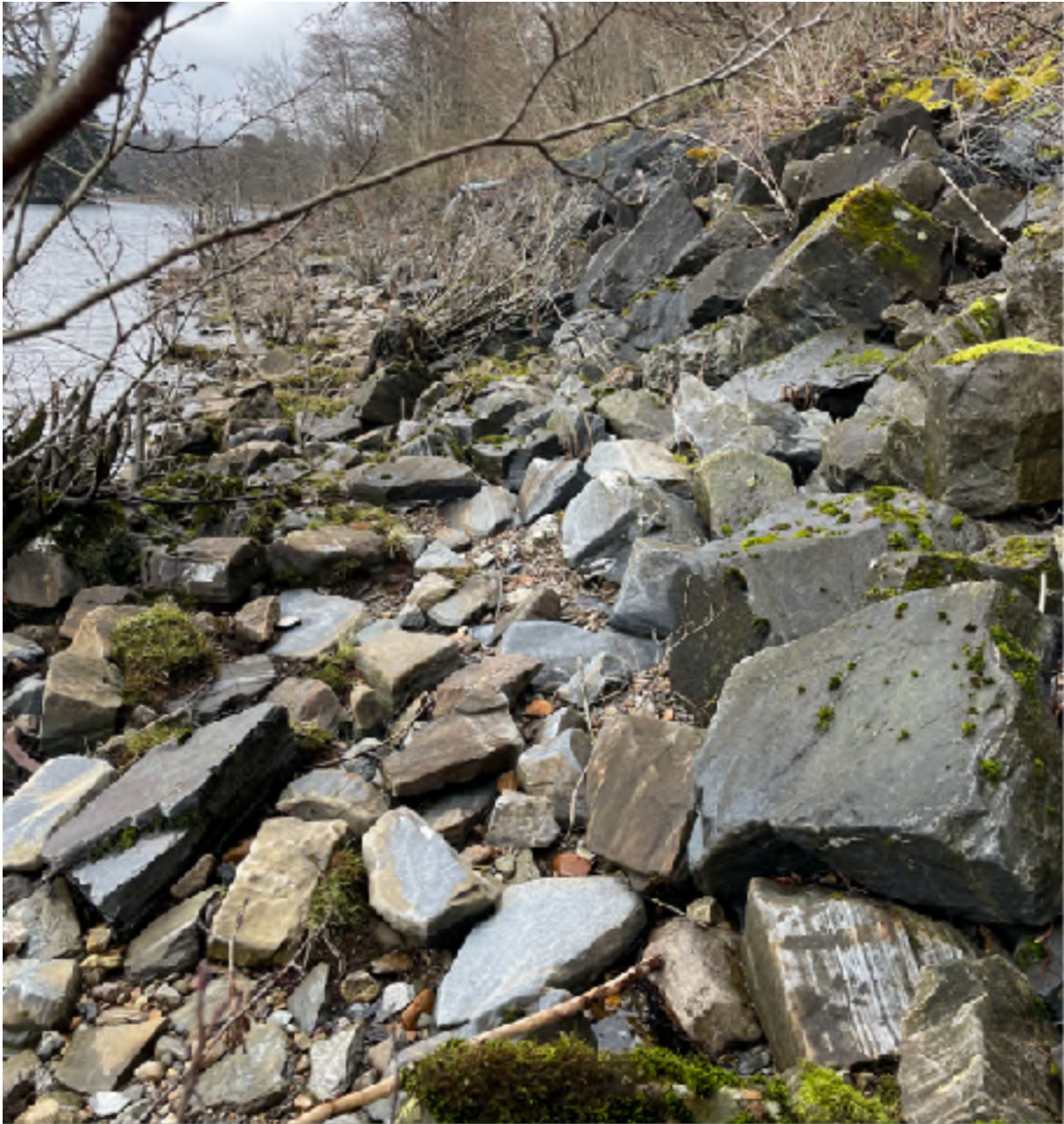
Armour rock foreshore protecting the road. Numerous large cavities between the rocks that could be used by otters.
