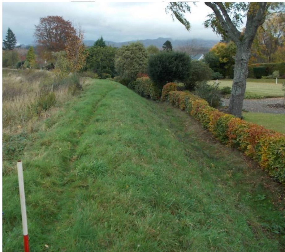
Photograph 2 – Localised bank erosion where bund changes direction
