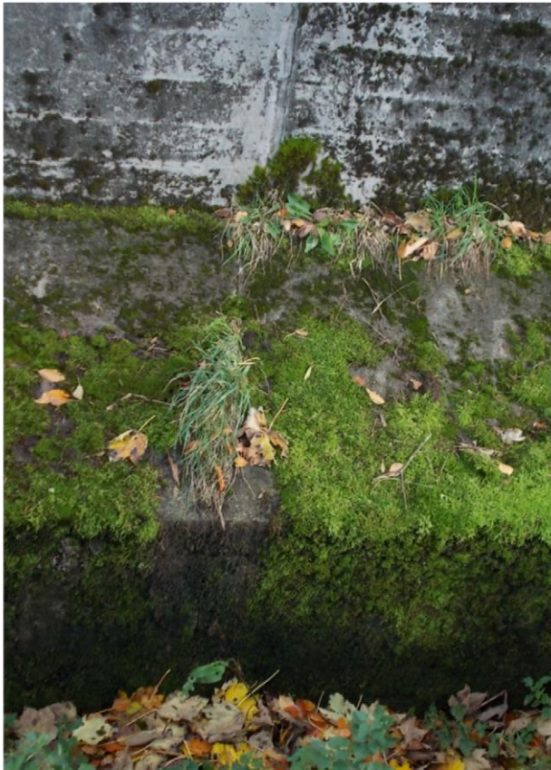
Photograph 19 wall cracked from top of wall to invert level
